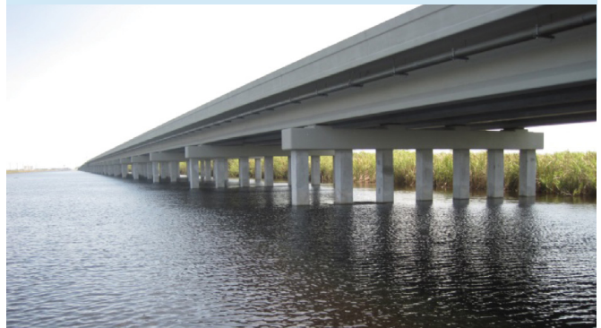
The 1-mile bridge along Tamiami Trail will help to restore flow into northeast Shark River Slough of Everglades National Park.
